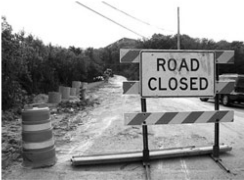
Lehman Road , constructed around the early 1800's, currently being improved along 1700 feet of roadway at a cost of $1.3 million.
